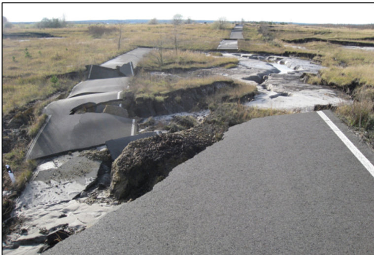
Figure 1: Example of a surface deformation (Photo; LMBV)
